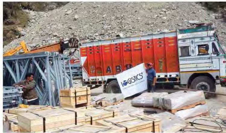
Logistics Plus India helped coordinate the replacement of a crucial bridge in the Himalayan mountains by moving parts to the installation site over some of the world's most challenging terrain.
