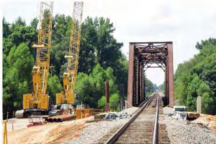
This through-truss bridge over South Carolina's Congaree River had to be replaced to allow clearance for the wide steam generator.
